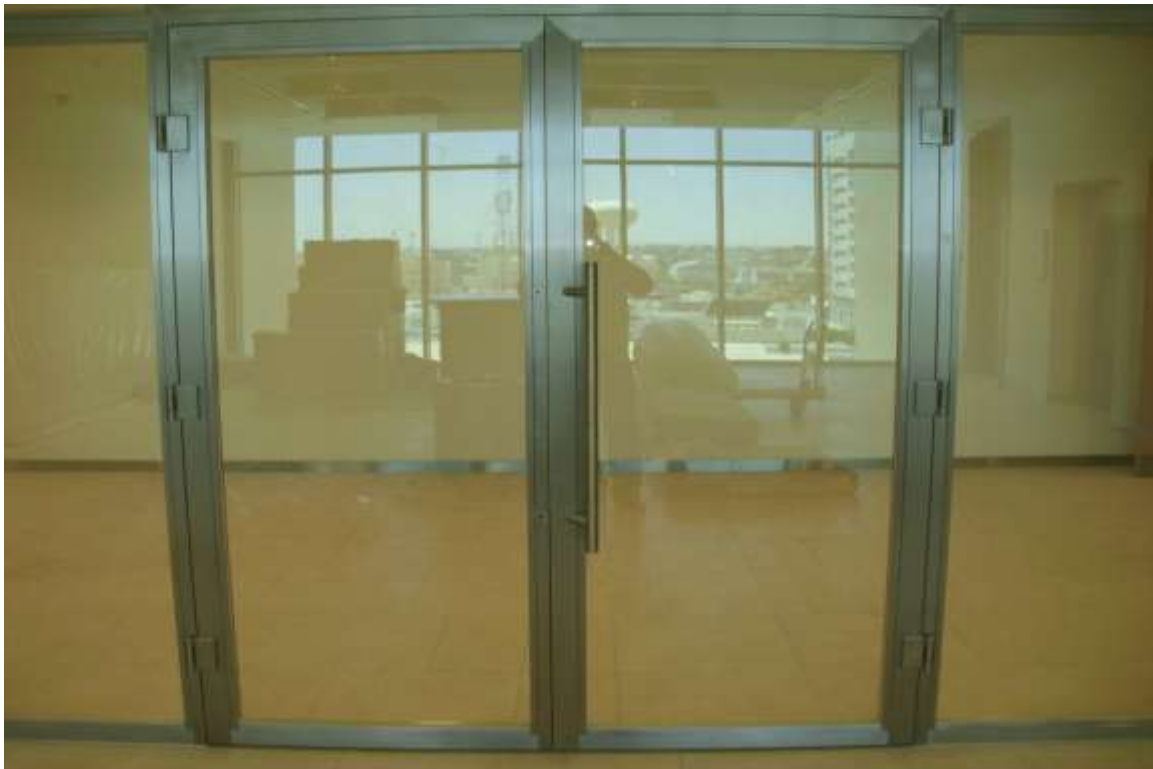
Fire Rated Door @ Survey & Land Registration Bureau - Kingdom of Bahrain.
